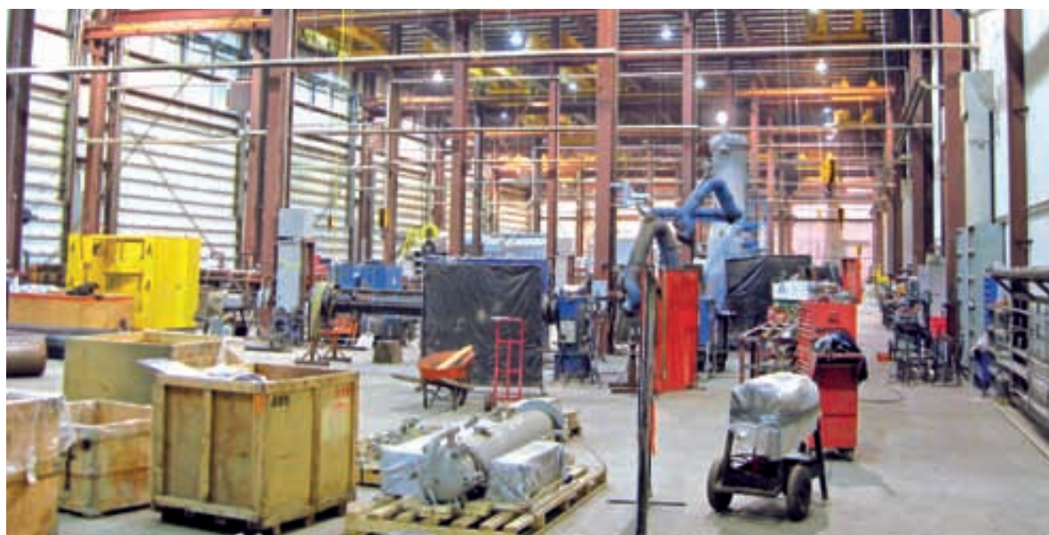
Once the wiring, PLC programming and plant commissioning is completed at the Enerflex factory, the entire skid is broken down into smaller sections for shipping
